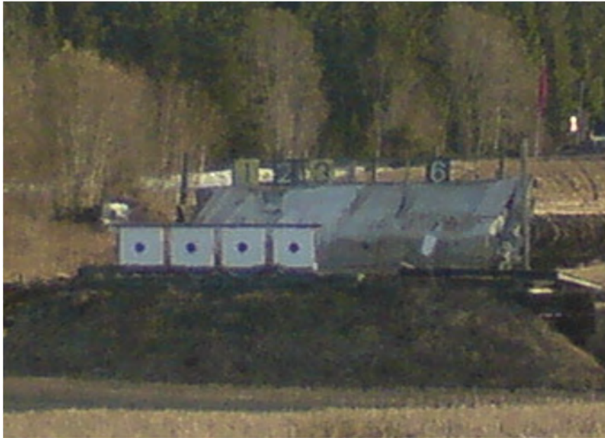
Figure 7 Bullet trap built up with a box of wooden poles and wooden beams
