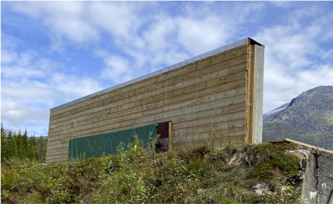
Figure 25 Bullet trap wall with interior vertical steel plate and a collection gutter for bullet fragments (the targets are covered by a green tarpaulin in the picture)
