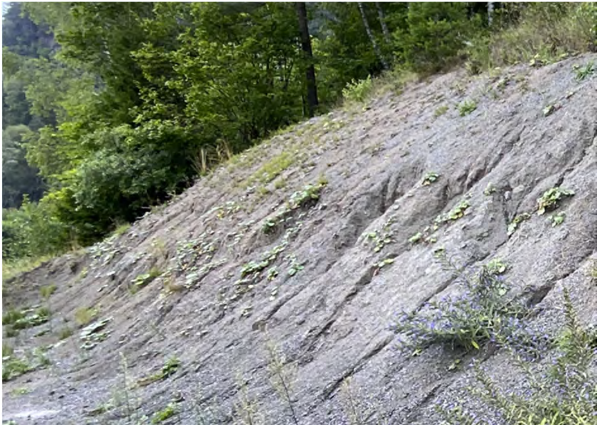
Figure 6 Example of crevice formation in a part of the bullet trap with fine gravel (foreground) and a lesser degree of crevice formation in a part of the bullet trap with soil (further away)
