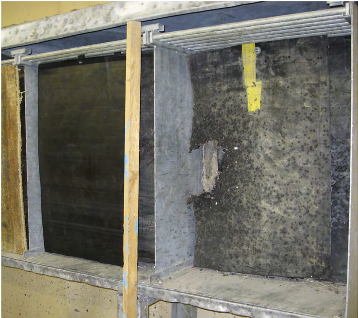
Figure 17 Steel box with vertical lamellas made of conveyor belts. Brünig Indoor in Switzerland
