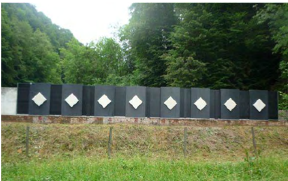
Figure 22 Bullet trap cassettes lined with steel plates. Leu + Helfenstein AG (Switzerland)
